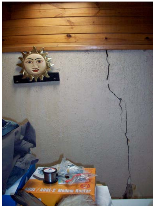
Figure 2. Cracks letting in cold air
