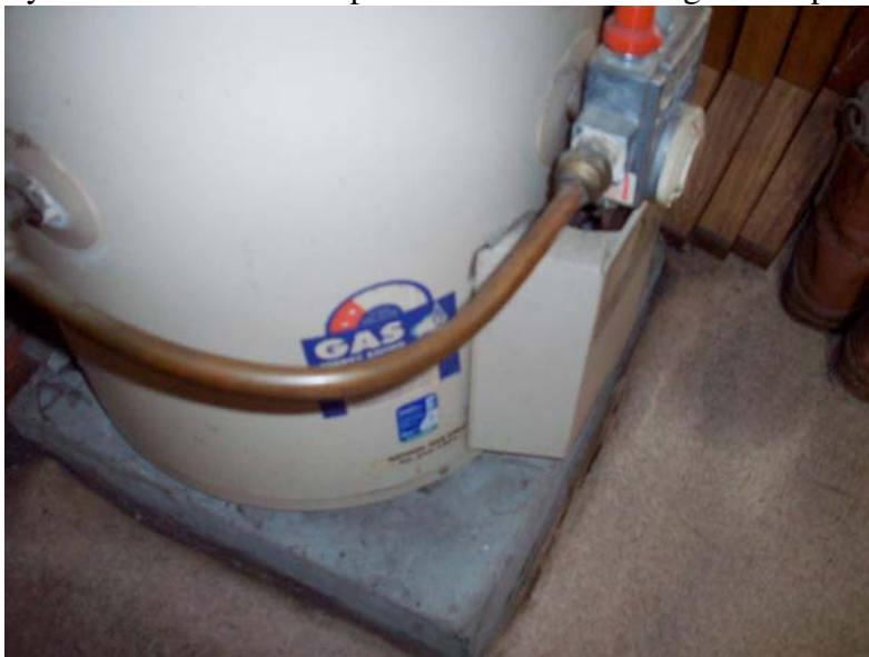
Figure 1. Our current hot water heater – note the 2 stars rating
