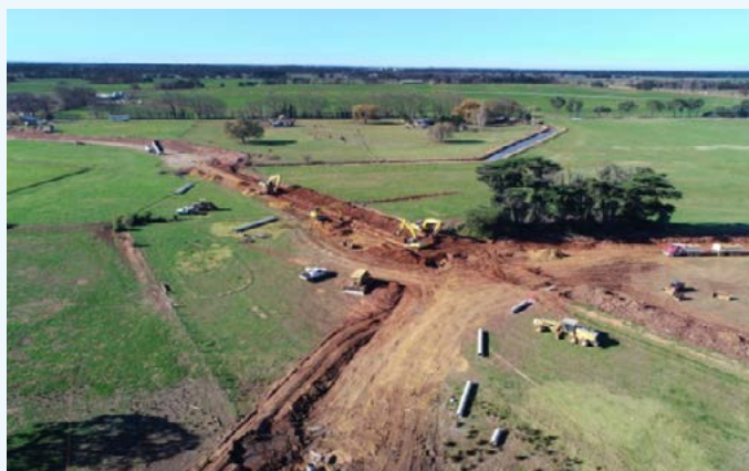
Figure 15: Modernisation works in the Macalister Irrigation District (courtesy of Southern Rural Water)
